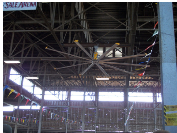
Both people and pigs in the Swine Barn at the 2011 Missouri State Fair will enjoy cooler conditions thanks to the installation of a new 24-foot fan above the show ring.
